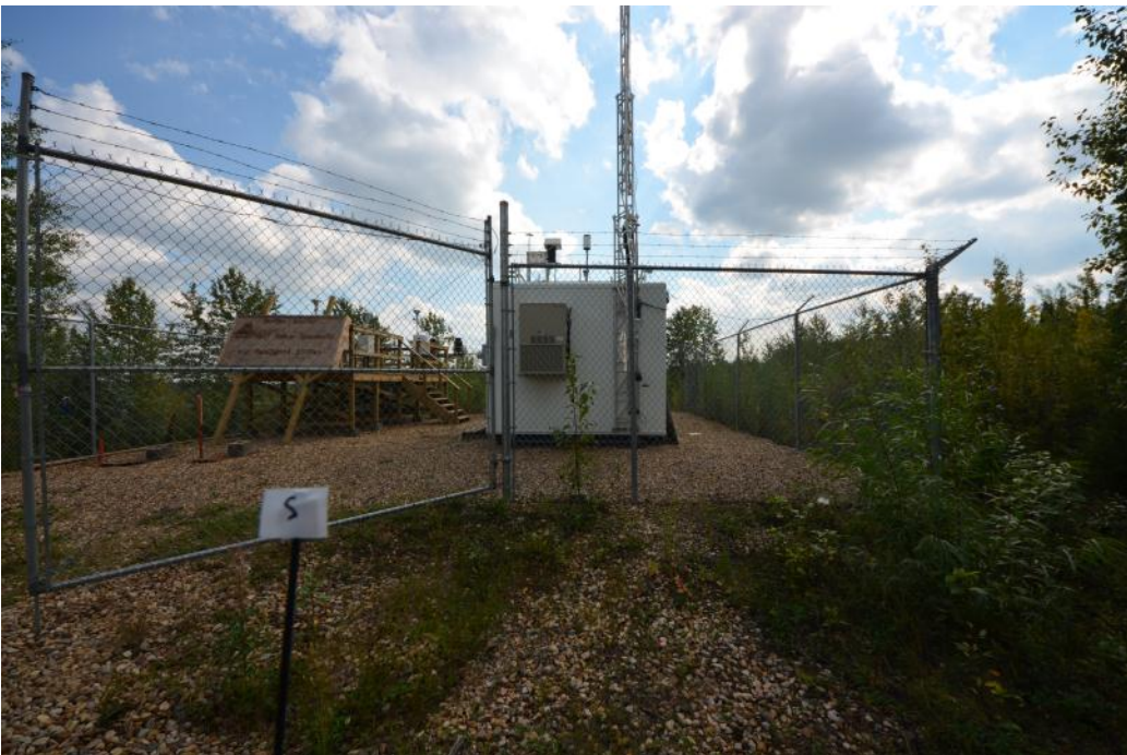
Figure 4.1 – monitoring compound looking south
