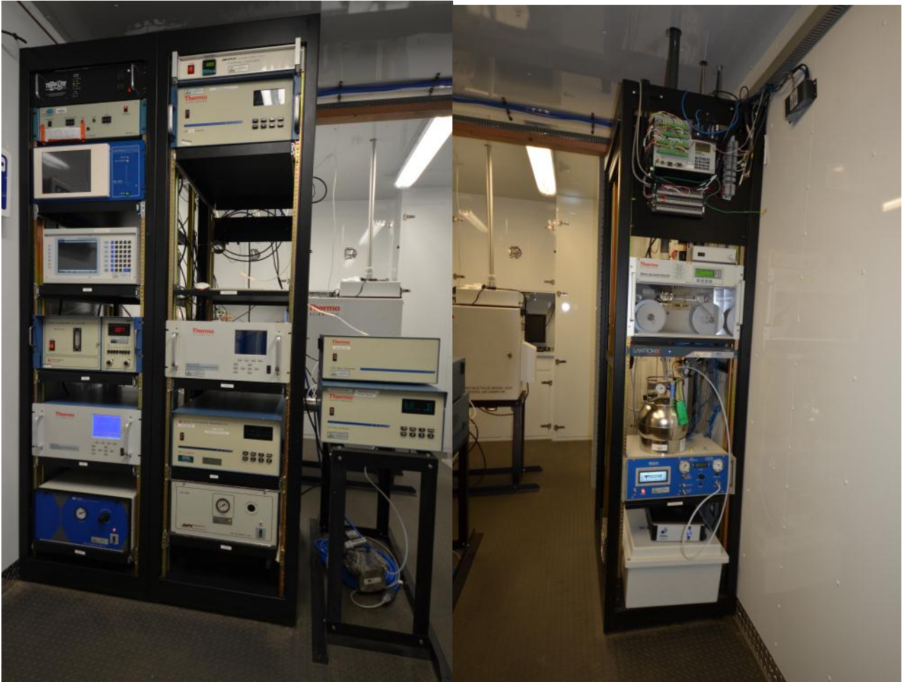
Figure 4.11 – East Rack (on the left) & West Rack
