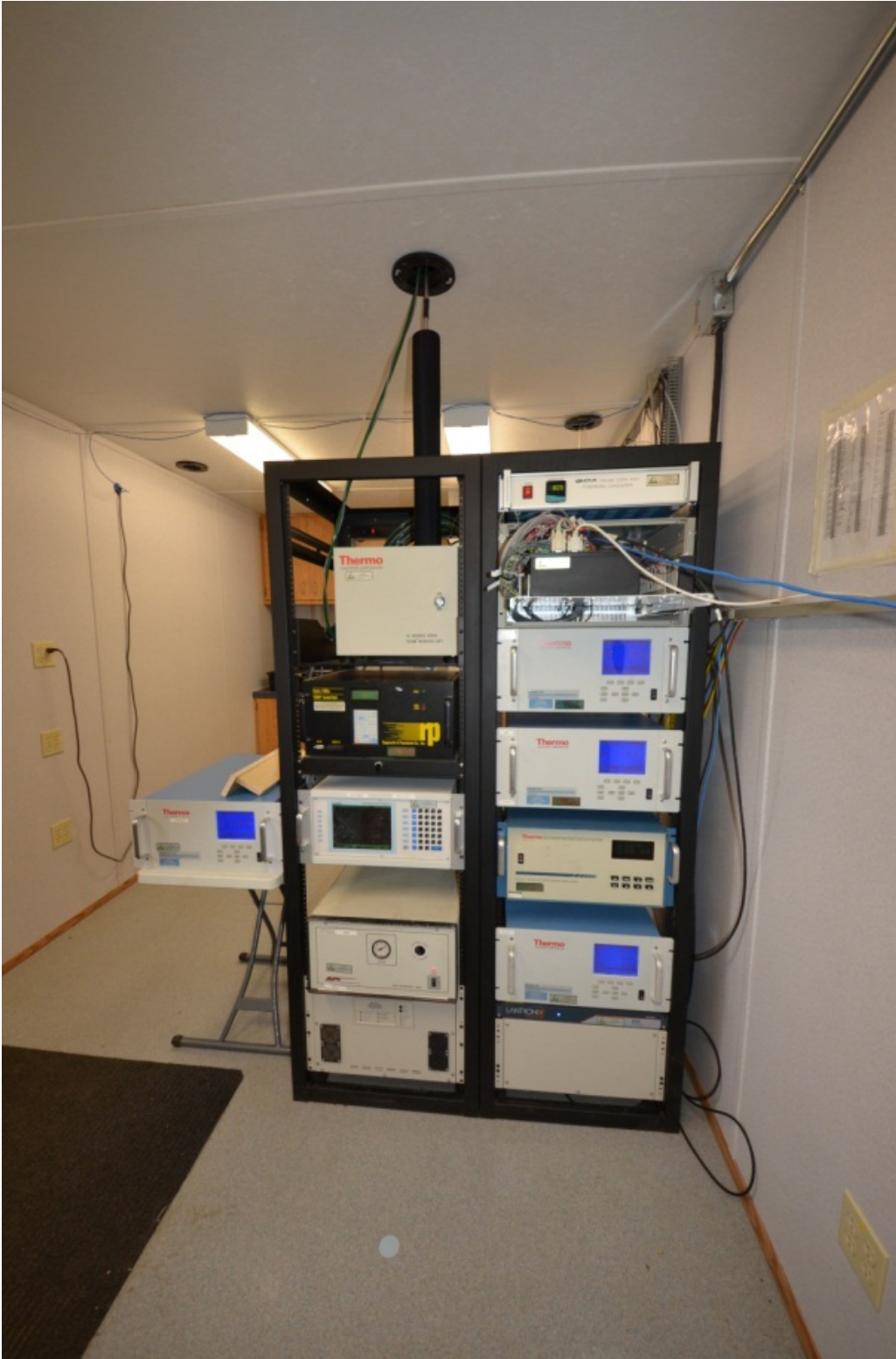
Figure 4.11 – East Rack (on the left) & West Rack
