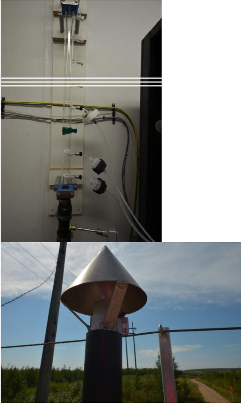
Figure 4.6 – Outdoor Sample Inlet & Indoor Sample Manifold
