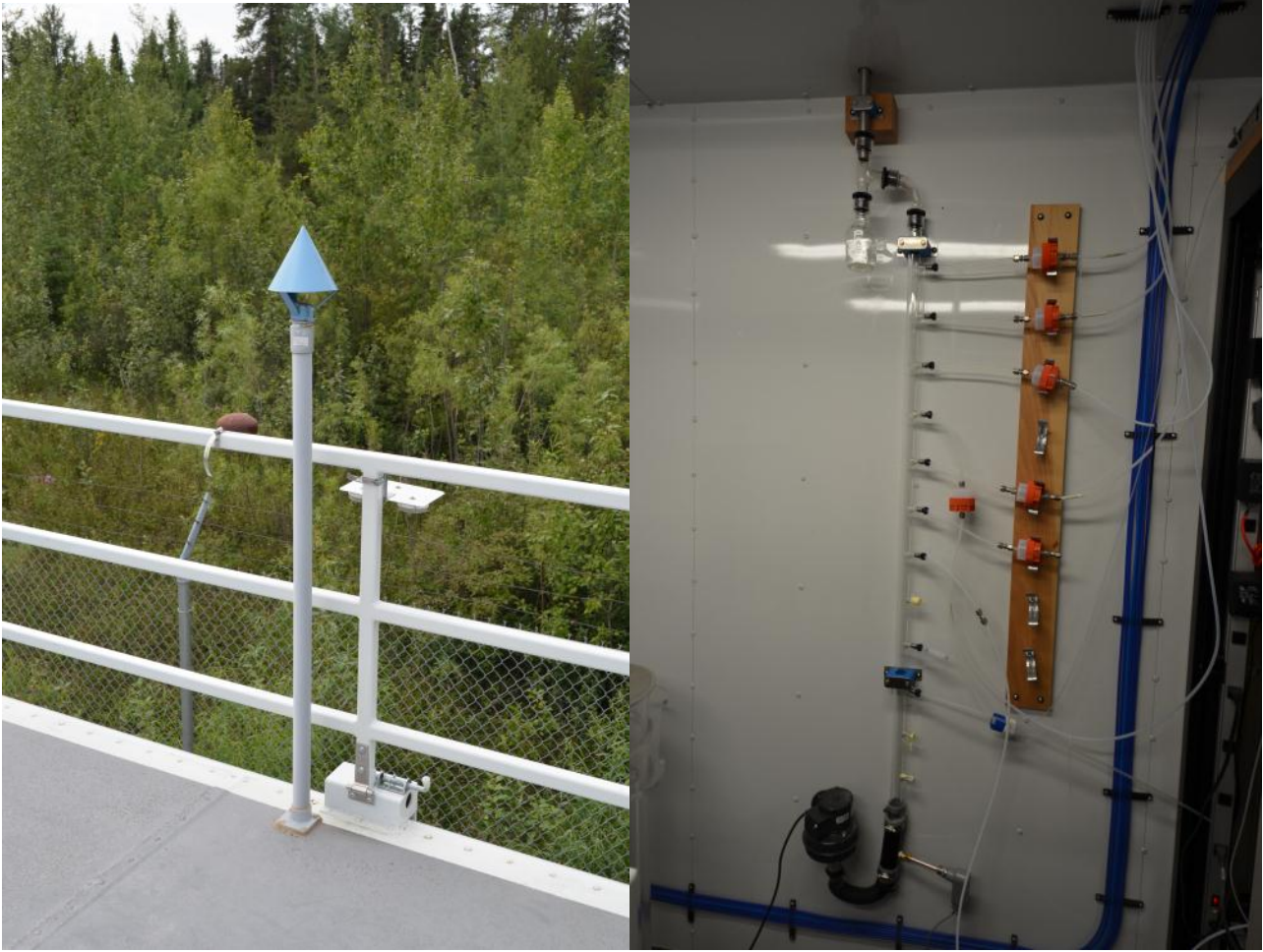
Figure 4.10 – Outdoor Sample Inlet & Indoor Sample Manifold
