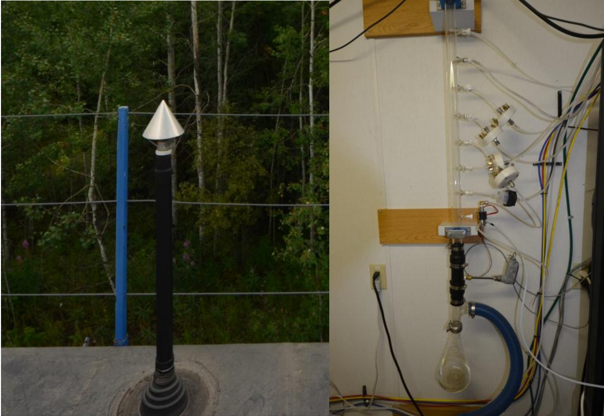
Figure 4.6 – Outdoor Sample Inlet & Indoor Sample Manifold
