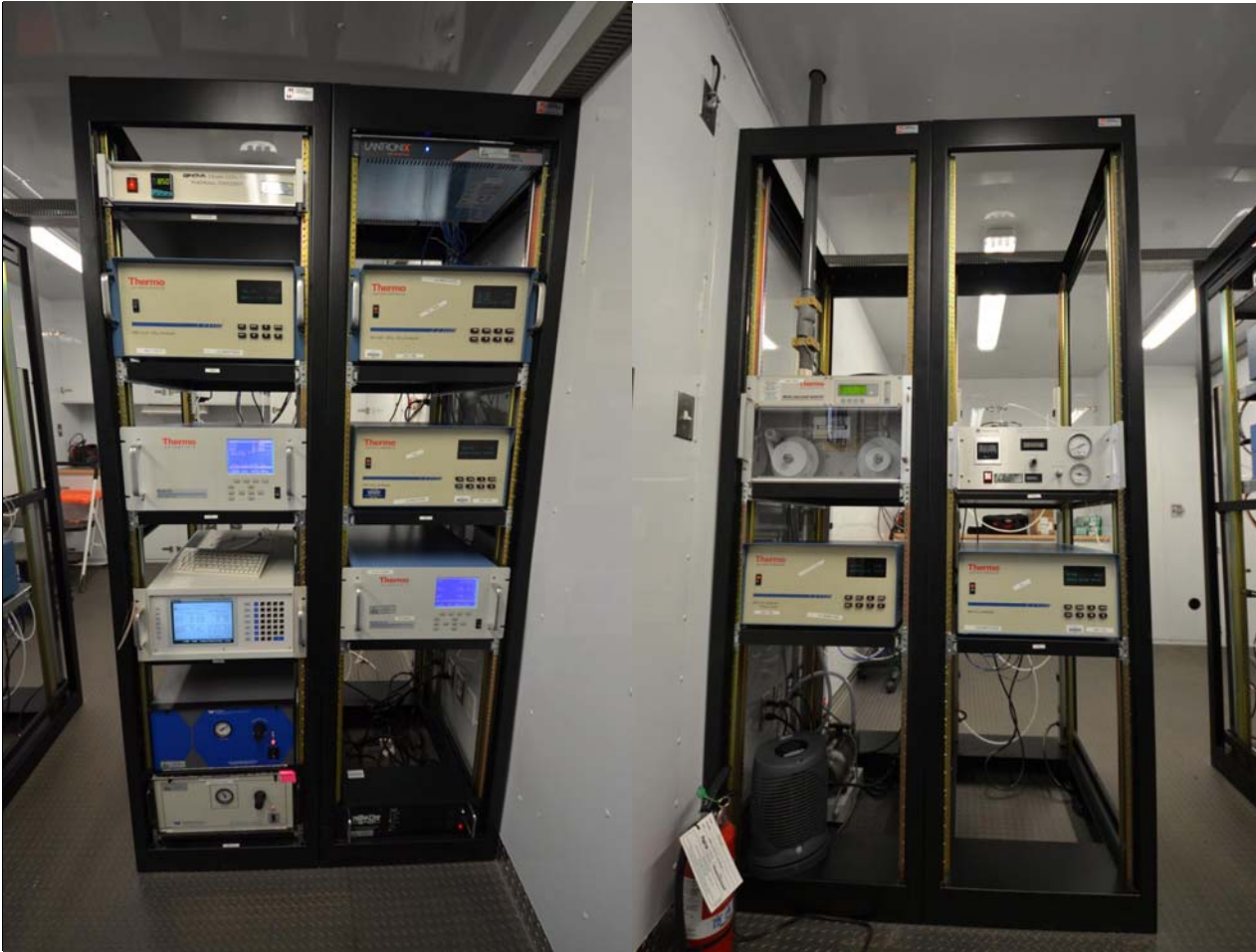
Figure 4.11 – East Rack (on the left) & West Rack
