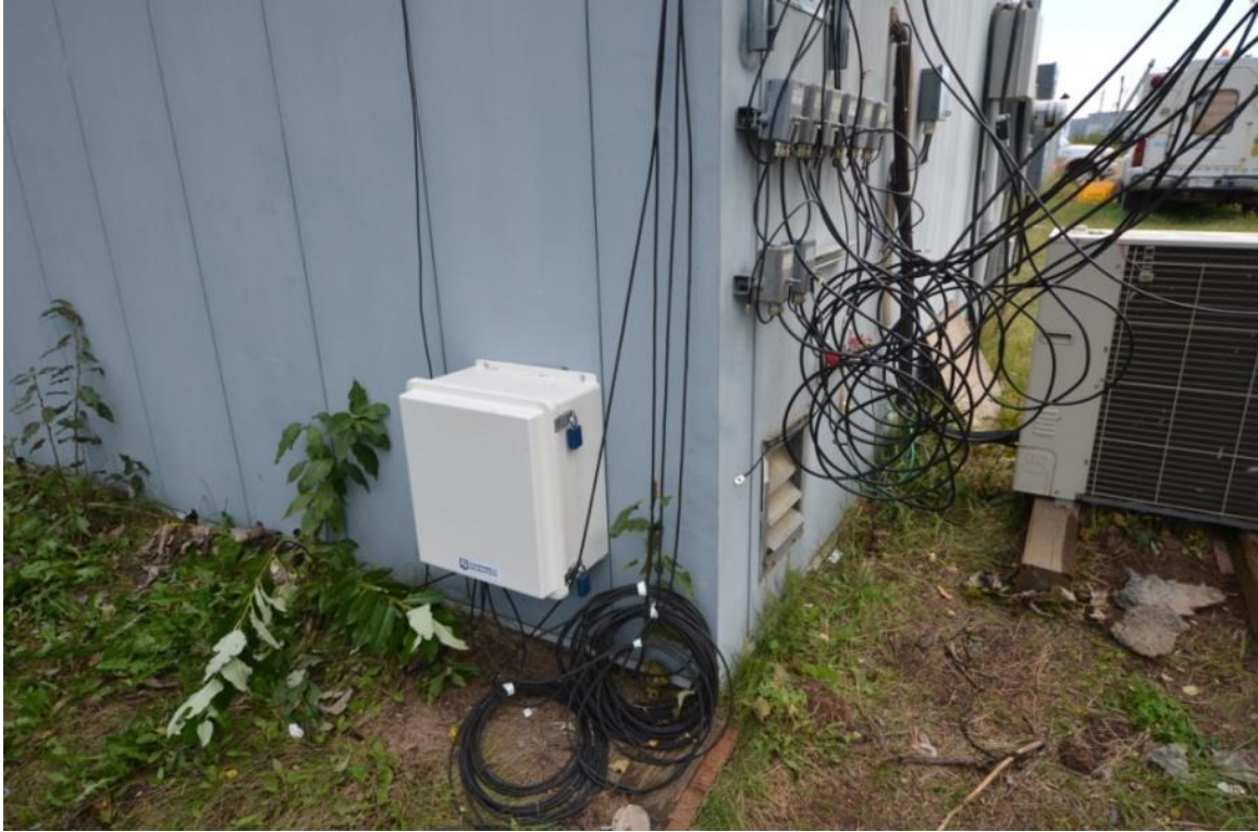
Figure 4.11 –Tower Data Logger
