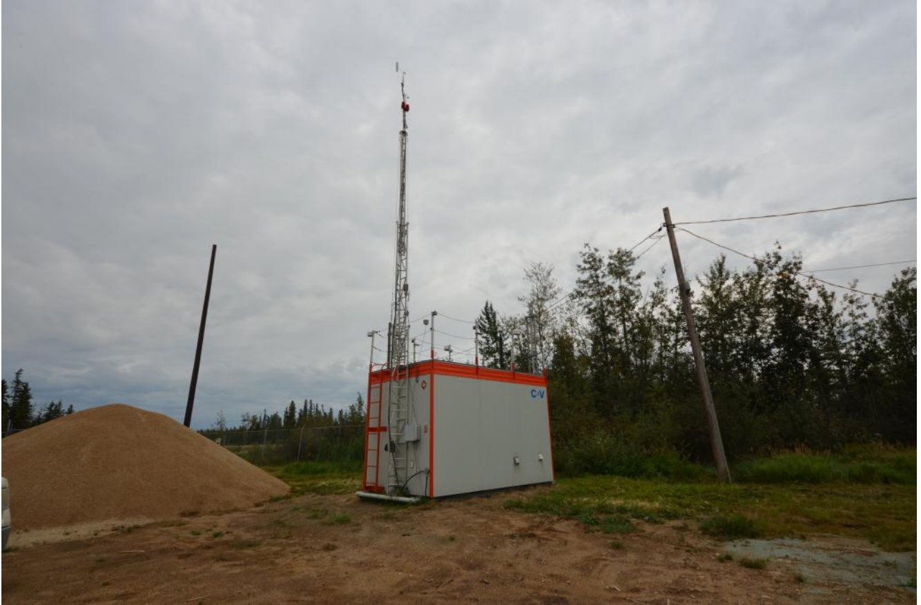
Figure 4.1 – monitoring compound looking south
