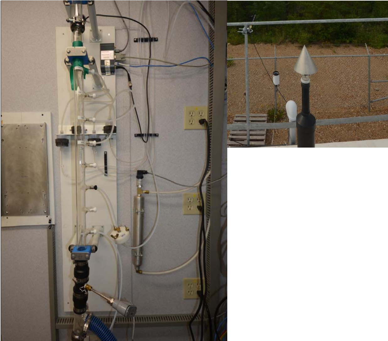
Figure 4.10 – Outdoor Sample Inlet & Indoor Sample Manifold
