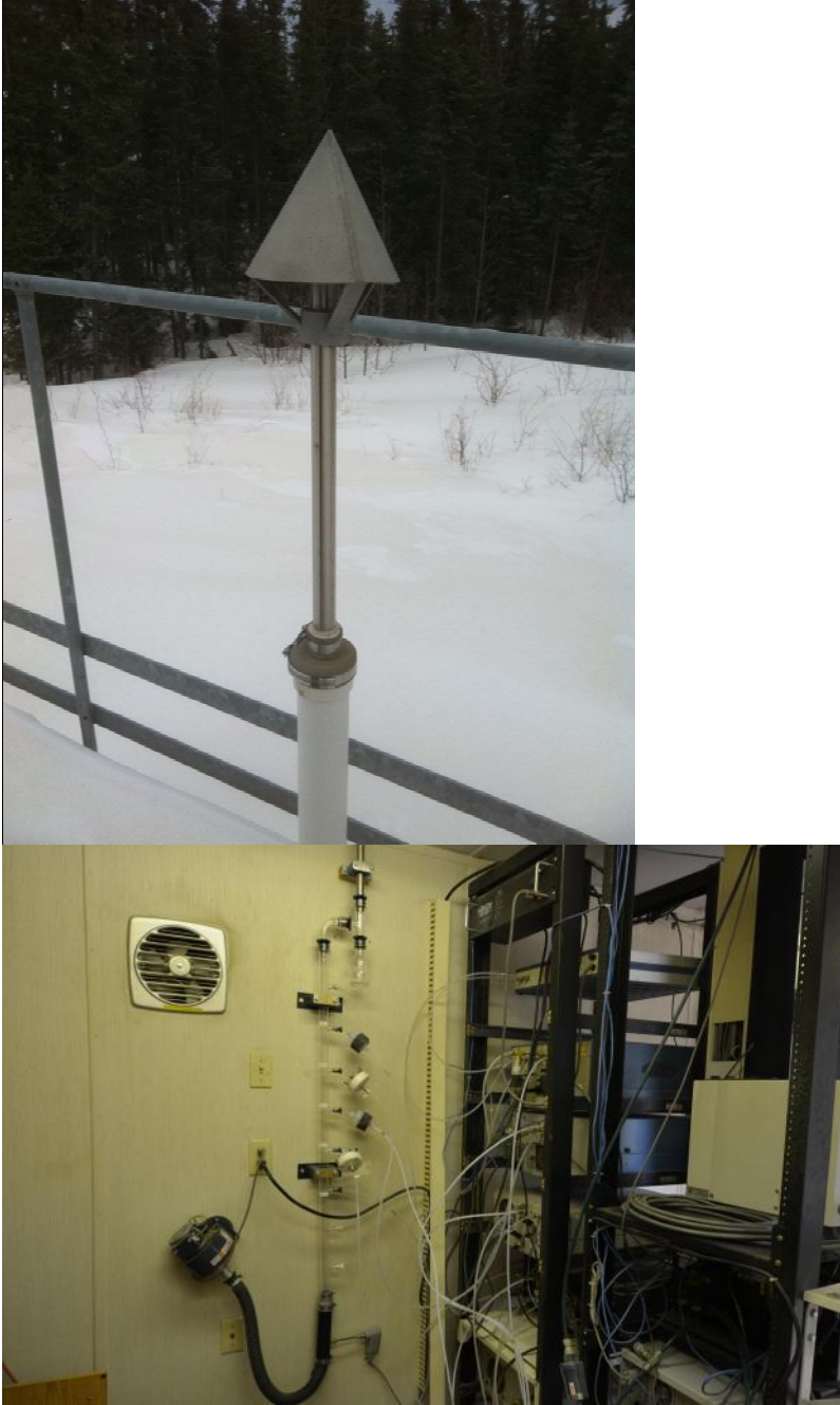
Figure 4.7 – Outdoor Sample Inlet & Indoor Sample Manifold
