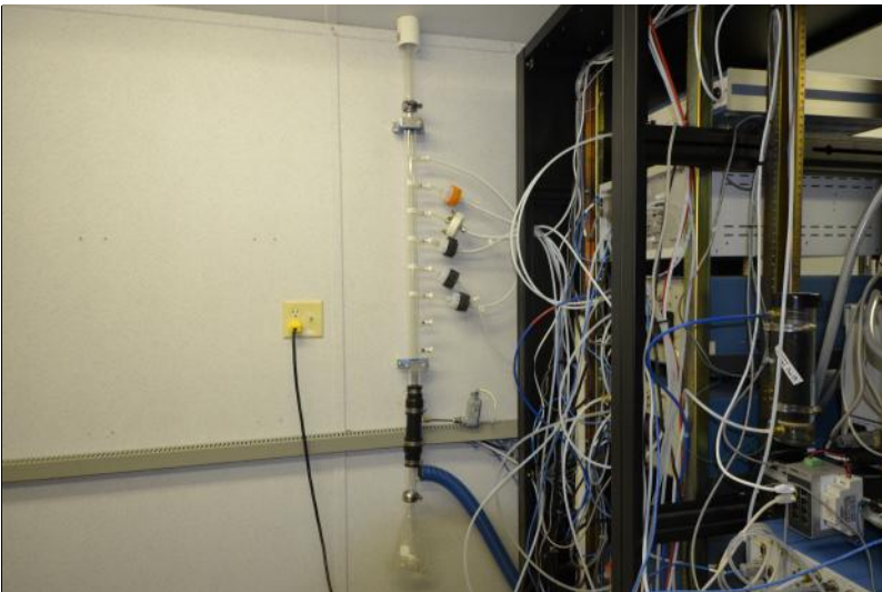
Figure 4.10 – Outdoor Sample Inlet & Indoor Sample Manifold
